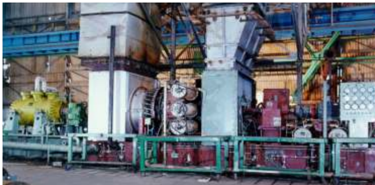
String test of gas turbine driven light end fractions compressor for Vijaipur
