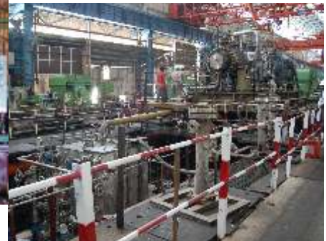
String test of motor driven compressor along with job lube oil system
