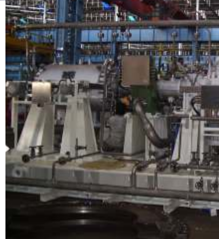
CO2 compressor train for a fertiliser plant in France
