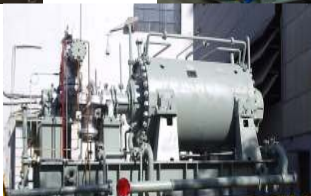
Steam turbine driven H2 Recycle gas compressor for motor spirit quality upgradation
