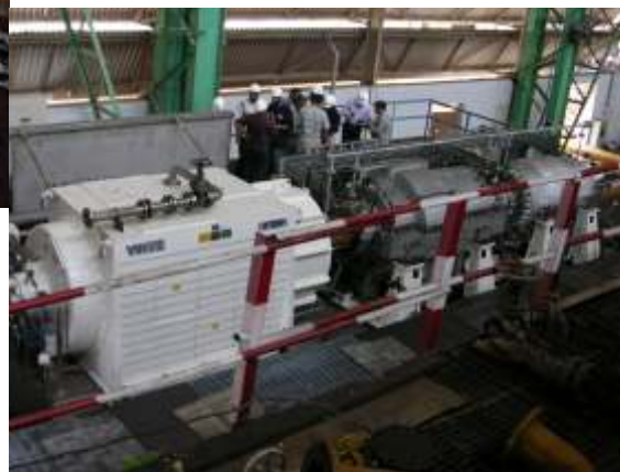
String test of Gas Lift Compressor train driven by motor for Lekhwair, Oman
