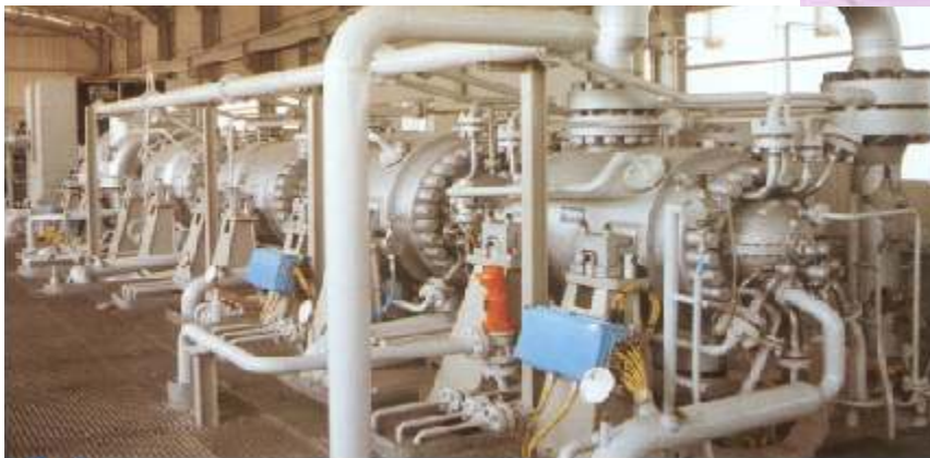
4 casing Synthesis gas compressor train in a fertiliser plant
