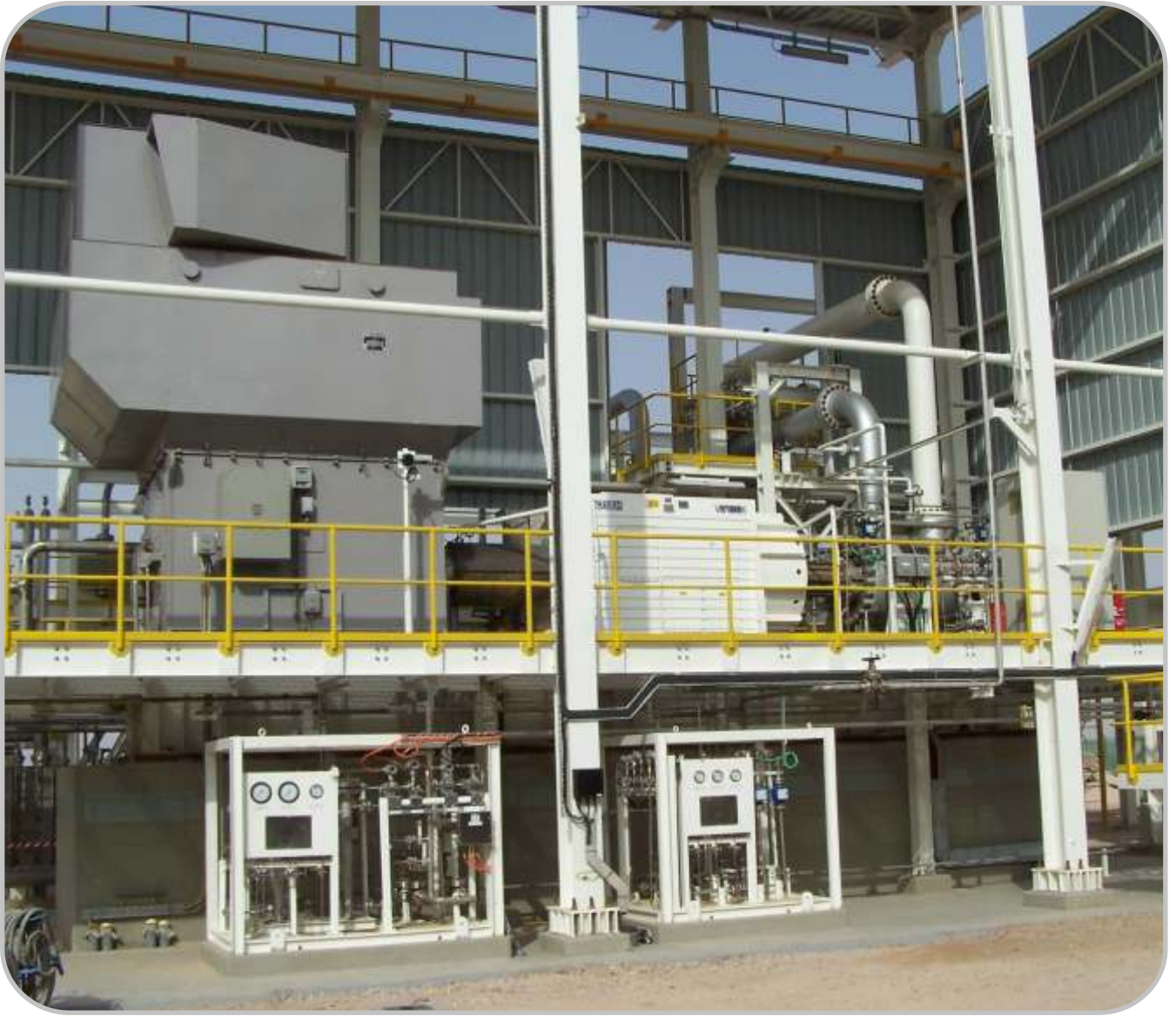
Depletion Compressor installed at Oman
